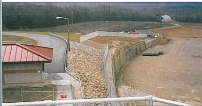
An installation for the U.S. Army Corps of Engineers at the Auxiliary Gated Spillway at Table Rock Lake in Branson, Missouri, included 1,600 feet of ornamental steel and approximately 1,300 feet of chain link fence on especially tough terrain.
