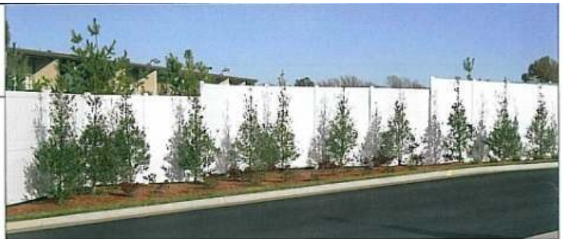
The company installed 2,185 feet of 12' Vinyl privacy fencing at the Oasis Inn
